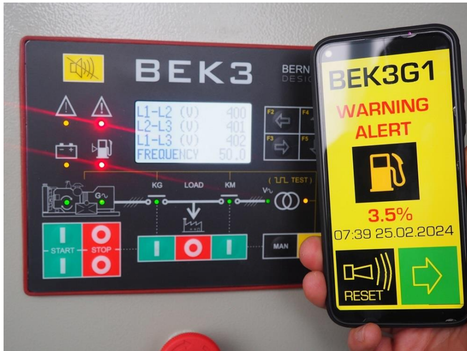
The BEK3 Automatic Transfer Switch Controller
